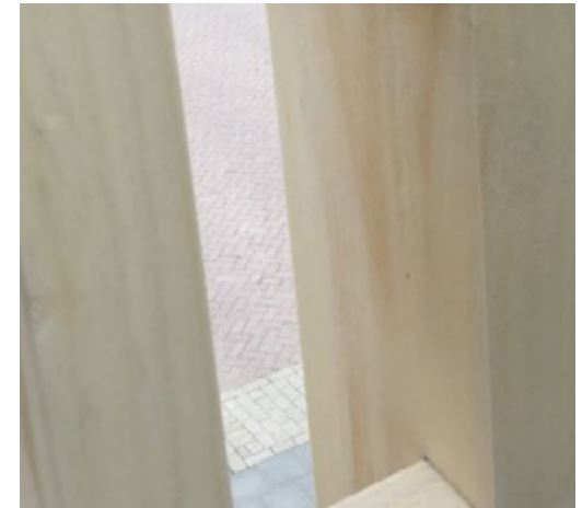
8.5 Reddish brown staining
